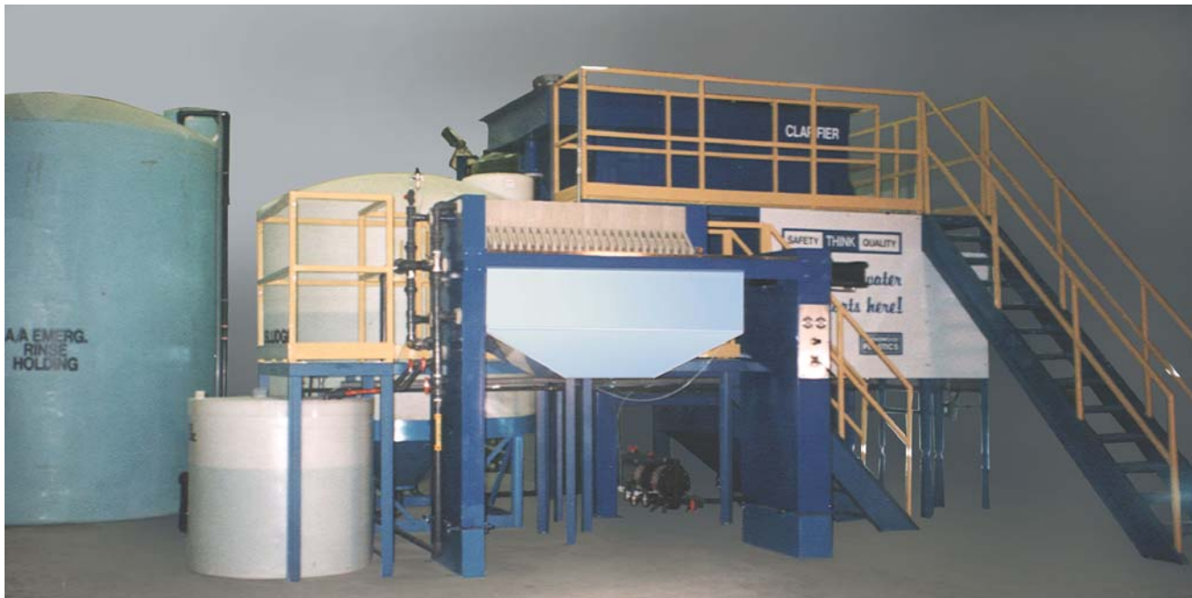
6391: Waste Water Treatment System
